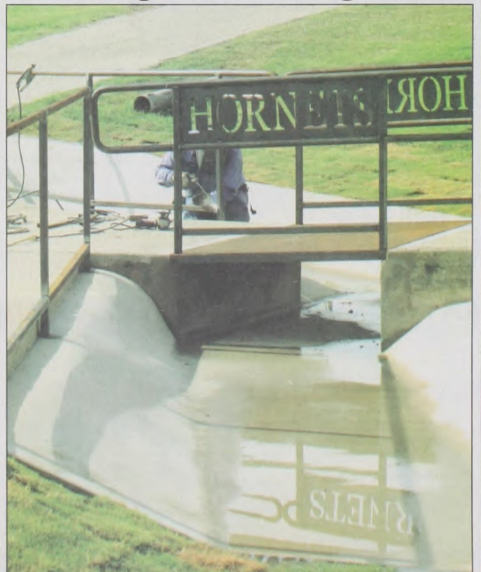
Neal Flusche of Flusche Enterprises welds railing over the drainage ditch in Hornet Stadium. Muenster ISD has had a drainage issue at the stadium, and with the additional water run off from the new cafeteria building, the District reconstructed the area to make the water drain better. Janie Hartman photo
