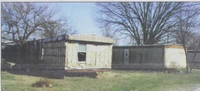
In Sylvan's Trailer Park, these two abandoned mobile homes and two more similar to them have been declared dangerous structures. Steps are being taken by the City to have them removed from the property. Three of the four were abandoned by their owners. Some have unsecured points of entry such as open windows. Janie Hartman photo
