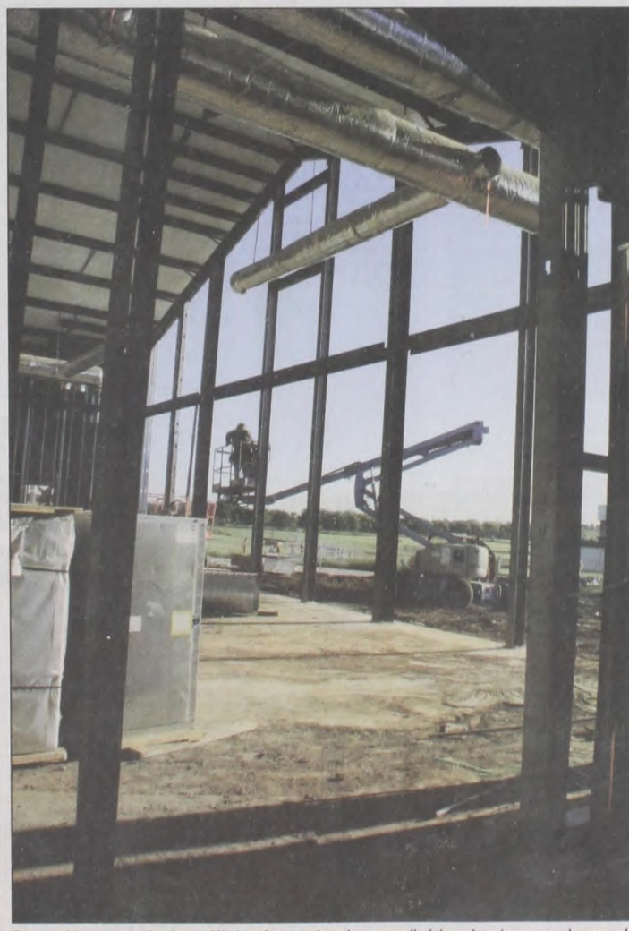
One outside area remained open Wednesday morning, the east wall of the cafeteria, as work proceeds on the construction of the addition to the Muenster High School building. Janie Hartman photo
