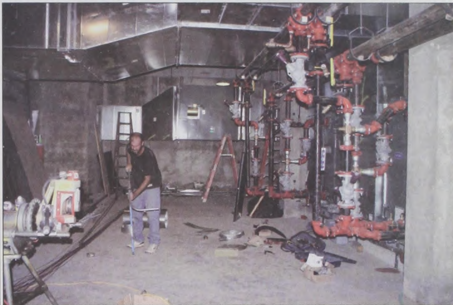
Workers from James Lane Air Conditioning and RMI Electric (above) continue the installation of the new heating/air conditioner/ventilation system in Sacred Heart Catholic Church. The new equipment and large air ducts are filling the basement of the church. Services will continue to be held in the Sacred Heart Community Center until the job is complete. Janie Hartman photo
