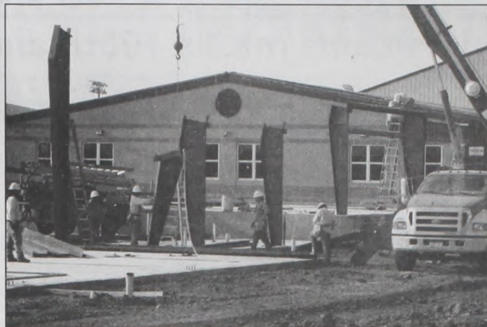
More than just dirt work can be seen on the Muenster ISD campus, as the first pillars went up Tuesday morning in the District's cafetorium building project. Janie Hartman photo
