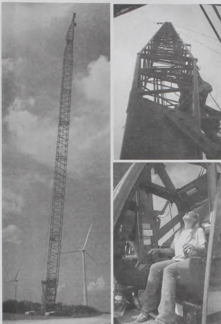
The crane operated by the Dillardards stands tall above the wind generators in the background. The tower to the right (#8) was the last to be installed at Wolf Ridge. Pictured lower right - Laurie Dillard sits at the controls looking up the long crane. Her view is shown in the upper picture.
