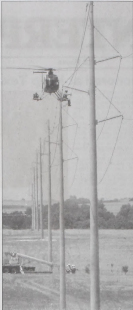
Florida Power and Light had Air2 install bird diverters onto power lines connected with the Wolf Ridge Wind project. FPL, an environmentally conscientious company, identified the area as the outskirts of a possible crane migration path. The devices make the wires more visible to keep birds from running into them. This line runs along CR 351. Janie Hartman photo
