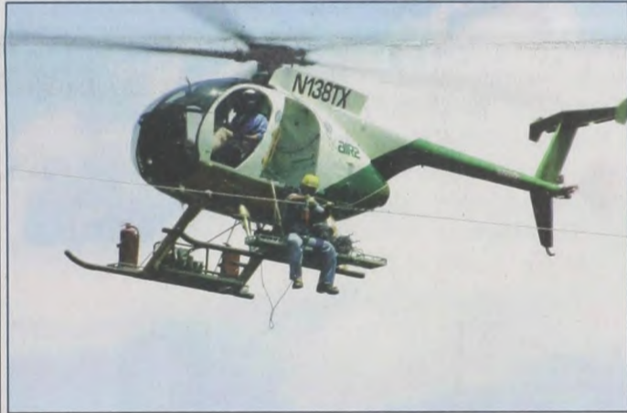
On Tuesday, crew from Air2, out of Timonium, Maryland, tied on "bird divertors" to the new electric lines recently installed northwest of town. The power lines will connect future electricity generated by Wolf Ridge wind turbines to a sub station west of town. Crew members were Jonathan Sole from Colorado, Todd Hooks from Florida, and Chris Jones from Alabama. Janie Hartman photo
