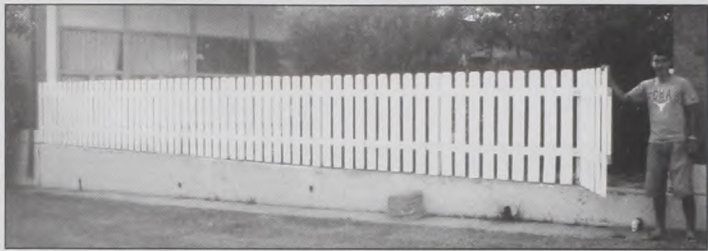
Brad Endres installed this fence between the MMH south parking lot and a courtyard of the patient patio. A locking gate allows for access with lawn equipment. Courtesy photo
