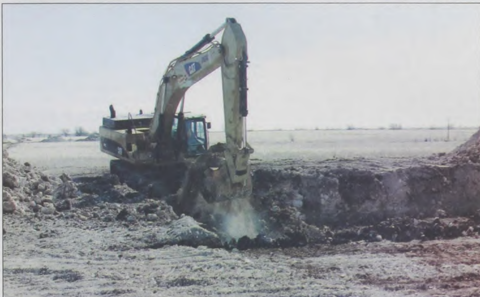
With an anticipated completion date of Oct. 1, preparation work has been progressing quickly for the Wolf Ridge Wind Project north of Muenster. This excavator operator digs dirt and rock from this hole
