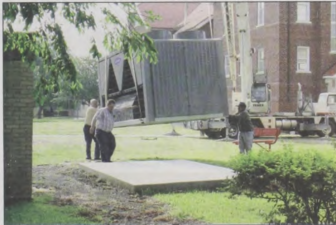
The new air conditioning unit for Sacred Heart Church arrived Wednesday morning and was placed on a pad north of the Church, with the assistance of Ernie Martin and Paul Fleitman. Major construction will begin Monday, June 23, which will cause the closing of the Church until the AC is back and running. Weekend services will be held in the Sacred Heart Community Center during construction. Janie Hartman photo
