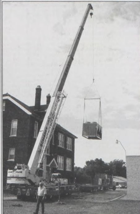
A large crane lifted a new air conditioning unit off the delivery truck and onto Sacred Heart Parish grounds Wednesday morning. Less "heated" services will be available in Sacred Heart Church later this summer. Janie Hartman photo
