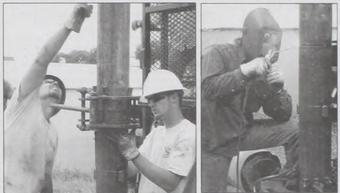
Muenster City Well #1 will soon be back in operation after workers put a steel liner inside the existing casing to eliminate a leak caused by a hole in the casing. The well has been shut down about a month. B&W Water Well Service pulled the well. In above photo, Corey Conrad and Rolan Jowell hook up a new joint. Below left, Jowell and Chad O'Dell line up the joints, so Jeff Solley of Reed's Welding (below right) can permanently attach the joints. Janie Hartman photos
