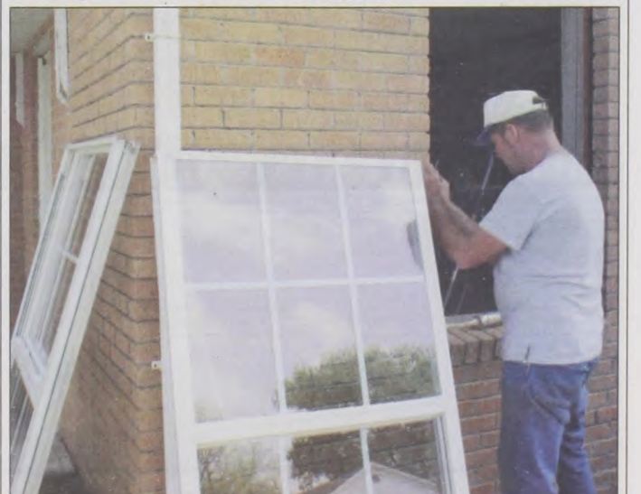
Don Eckart of Eckart Construction replaces one of all but three windows at the First Baptist Church. Other improvements being done include a new roof and replacing two exterior doors. The "hall" of the Church was built over 50 years ago, with the newer addition in the early 1980s. Janie Hartman photo
