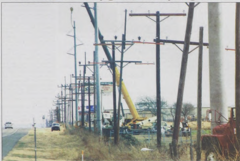
Rebuilding of electric lines along Hwy. 82 east of Muenster is Oncor Electric Delivery's current project in this area. The lines were originally installed in 1927 and updated in 1961, according to Sabrina Taylor, Oncor's area manager. They are replacing the old wooden poles with new poles, either of cement or steel, that will withstand the Texas weather, as well as present a more pleasant appearance. They are also putting up new conductor lines. There are 22 miles of poles and line slated for replacement. The designated lines run from the Muenster substation to Gainesville. Oncor plans to have 168 of the new cement and steel poles in place by April. Oncor contracted with Chapman Construction and Texas Electric to do the work on their behalf. Janie Hartman photo
