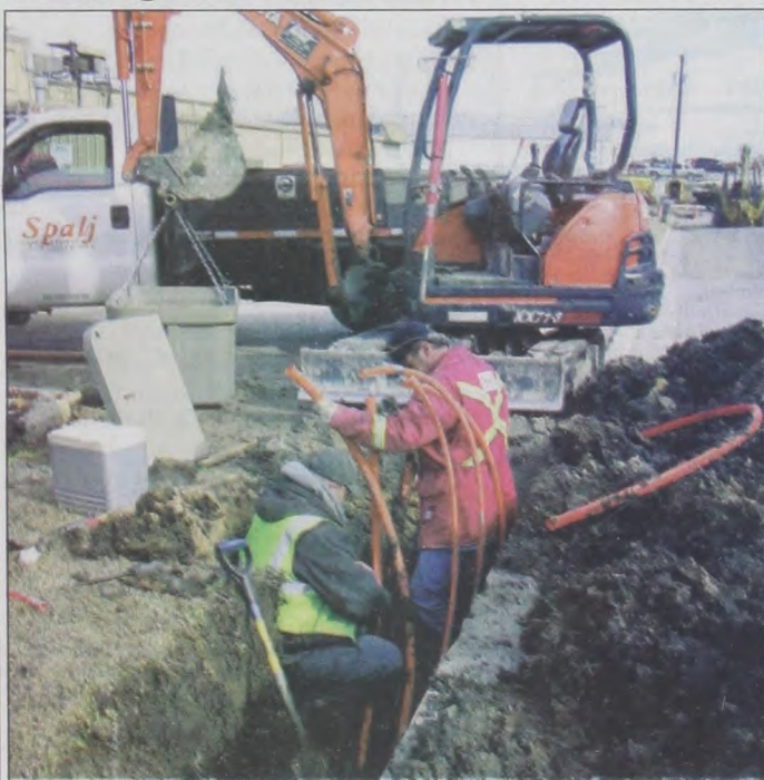
Jim Davis, top, and Carl Strom of Spalj install fiber-optic lines in Muenster for Nortex Communications. All of Nortex's above ground copper wiring for homes and businesses in Muenster and Valley View is being replaced with fiber-optic wiring. When completed, Nortex will be able to offer faster Internet service and more television channels to its customers. Completion is anticipated by this spring. Janie Hartman photo
