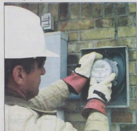
John Walterscheid of Cooke County Electric Cooperative (CCEC) installs a new Automatic Meter Reading (AMR) device. All members of CCEC will have the new meters installed during January and February. Courtesy photo
