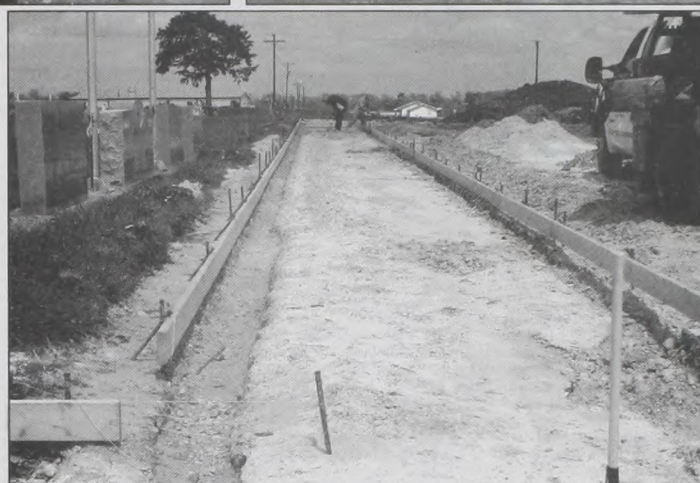
Construction continues on the extension of the 7th Street sidewalk from Sacred Heart Church to the cemetery. The new 8 foot walkway above is also being installed by Huchton Construction into the east side of the cemetery. Janie Hartman photo
