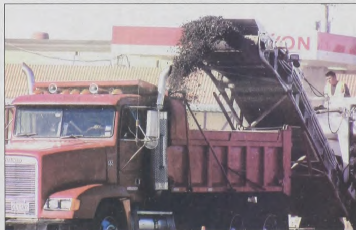
Work began Wednesday morning to repair Highway 82 through Muenster. The seal coat laid down last July was damaged when the tender coat got hot, causing the tar to bleed through, then was picked up by vehicles, making numerous holes and bumps. The old surface is being removed and a new, hopefully smooth finish should soon appear. Janie Hartman photo
