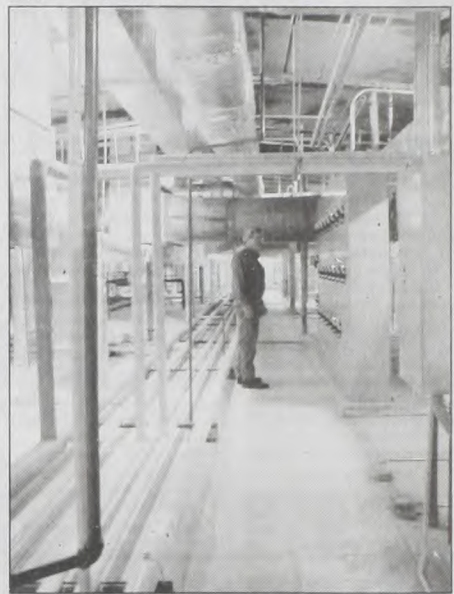
Above the Cooke County Justice Center in the mezzanine, lines and ducts necessary for daily operation of the facility fill the transfer room. Commissioner Al Smith examines the electrical transfer junction boxes. Turn off valves located above each inmate unit make it easy for jailers to turn off water if needed.
