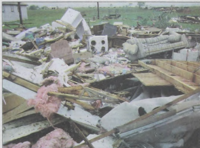
A mobile home and a camper trailer south of Lindsay were totally destroyed by strong winds. Shauner and James Shellhorn and their 3 children lived in the home owned by Ricky Pittner. Dan Martin, living in the trailer, also lost all his belongings. See page 4 for more storm pictures. Picture by Janie Hartman
