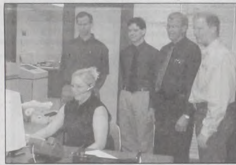
Malony Bartush, Cooke County Electric Co-op telephone/receptionist, tests the new Avaya phone system recently installed at CCEC. Also pictured are, from left, Neil Hesse, CCEC president, Chris McNamara, Nortek internet technician, Alvin Fuhrman, president and CEO of Nortek Communications, and Shane Wiley, CCEC office manager. Courtesy photo
