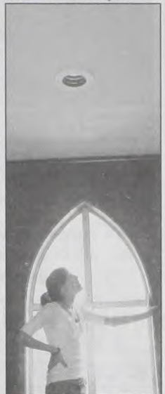
Mary Cochran stands framed in a window of the Sacred Heart Parish Sisters' Chapel. She is checking out the work done on the Chapel ceiling, which needed tiles replaced due to roof leakage. Janet Felderhoff photo
