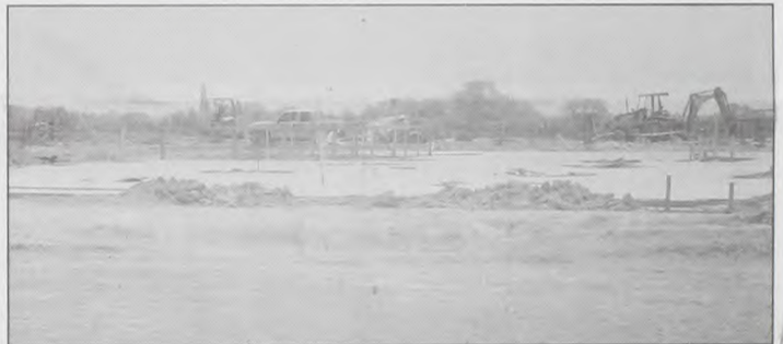
Construction of the new Cooke County Justice Center has been progressing for about a month and a half. The slab was poured this week. Sedalco Project Supervisor Bud Howard reports that about 25-40 workers are on the scene daily. This number will increase as the project gets further along.
