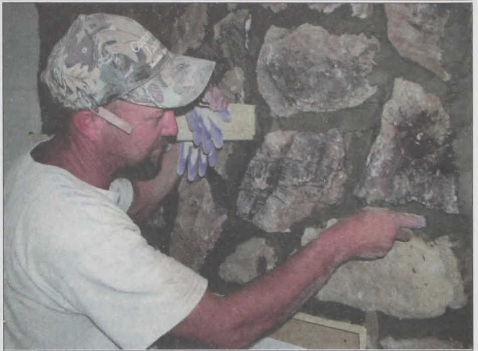
Mason David Hillard puts the finishing touches on a rock face fireplace. After arranging all of the stones on the wall, he cleans the surface to make it more attractive. Hillard is a mason who enjoys a creative challenge in his tile, stone, brick, or block work. Janie Hartman photo
