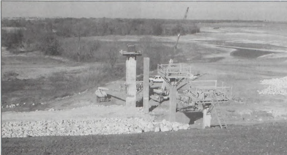
Dam construction at the Muenster Lake project is complete except for a little fill-in and vegetation, according to Raymond Lee, NRCS inspector, who also noted that the spillway is still under construction, but functional. Over 1,350,000 yards of dirt was used to build the dam. Pictured above, work continues on the gate valves that will draw water for the City at three different levels, as the last of the 19,000 tons of rock-rip-rap gets laid to protect the front sloop. In the background is the 308 acres that will one day be under water. This multi-purpose lake is financed in part by the Natural Resource Conservation Service and the Muenster Water Board as a watershed, flood control project. Janie Hartman photo
