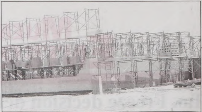
COOKE COUNTY JUSTICE CENTER - Construction of the new County Jail facility is progressing on schedule. Most of the slab has been poured with the exception of the kitchen area that is being plumbed. Block walls are going up. Janie Hartman photo
