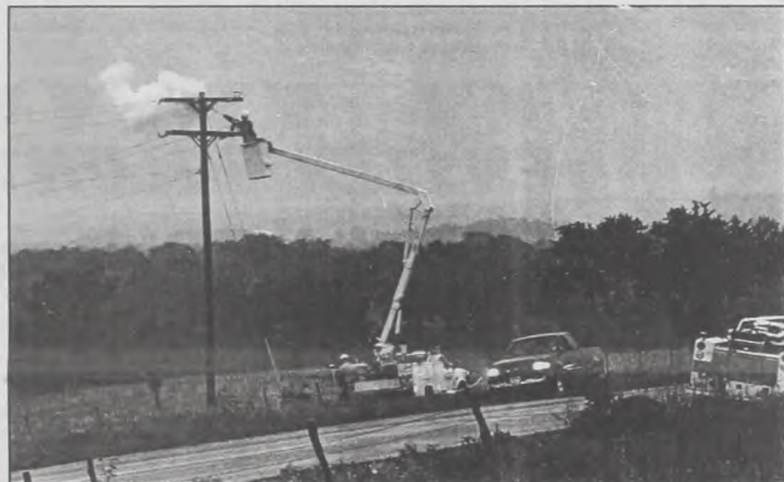
Cooke County Electric Cooperative employee Gary Growing extinguishes a small fire on the cross-arm at the top of a utility pole north of Muenster on FM. 373. The fire occurred around 11:00 a.m. Wednesday when an insulator failed. CCEC employee Bob Tamplin assisted Growing in replacing all six sets of the insulators on the pole. A 911 call to the Muenster VFD put them at the scene, but their assistance was not needed. Janie Hartman photo
