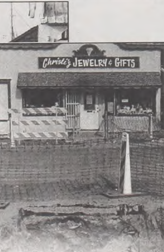
Muenster's second block of Main Street had concrete poured for curbs on Wednesday as part of the KMB Beautification project. Crews are show working in front of The Old Theatre Mall. At left - Christi's Jewelry and Gehrig's Hardware have had six foot holes bored in the ground in front of their buildings for several days. Customer traffic is slower in some businesses due to the construction. Christi's closed early a number of days. Janie Hartman photos
