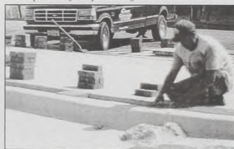
Workers put some finishing touches to the west side of Second Street this week, including decorative brick.
