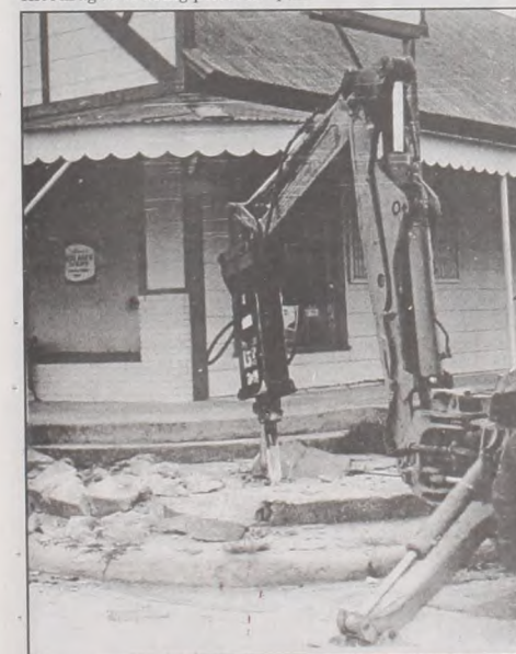
Reconstruction of the sidewalks on Main Street moved to the east side of Second Street this week as crews demolished and cleared the area of old concrete. Janie Hartman photo
