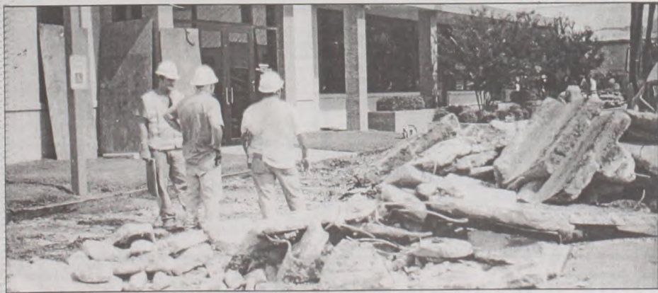
Work began last week on the Keep Muenster Beautiful Main Street project. Destruction started on the west side of the
