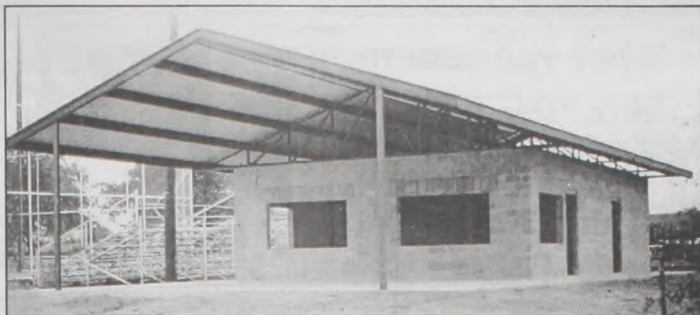
The Muenster Jaycees' progress continues at the Ball Park as the concession stand/bathroom building is being constructed. Janie Hartman photo
