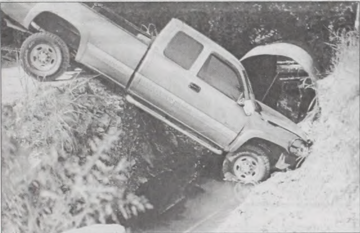
Neglecting to observe traffic warning signs could result in a situation similar to the one above. Rushing water pushed the 7 foot culvert out of CR 424 leaving a drop off of about 8 feet. The washed-out culvert is located on CR 424 east of Muenster near the Klement Dairy. See pg. 2 photo of second road barricade that was disregarded by the trio involved in this incident.
