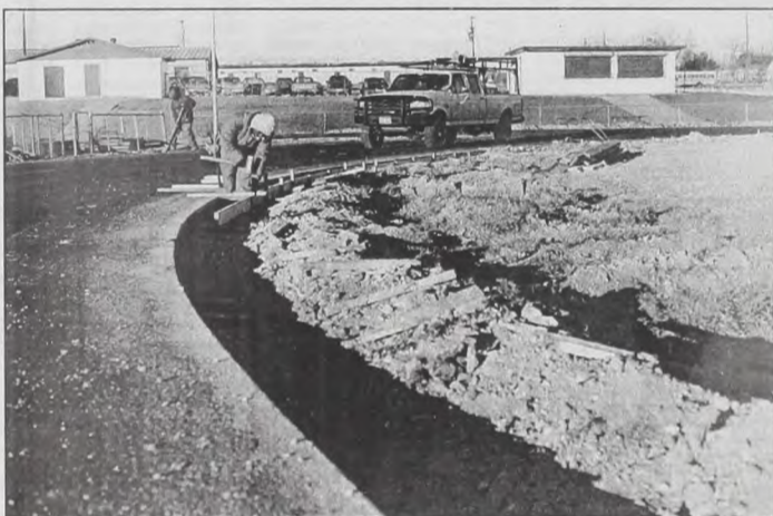
Work has begun on a Muenster ISD track. Workers are building a new curb, then will resurface the track. Photo by Janie Hartman
