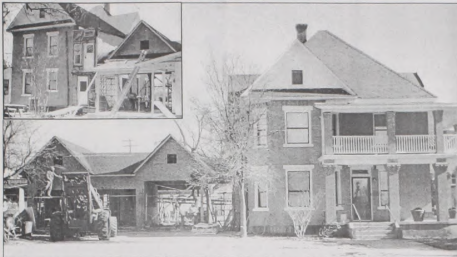
Progress continues on the Sacred Heart Rectory, as the original 1907 building gets a face lift and the new garage/shop addition gets covered. The inset picture shows the back (east) side of the project. Janie Hartman photo
