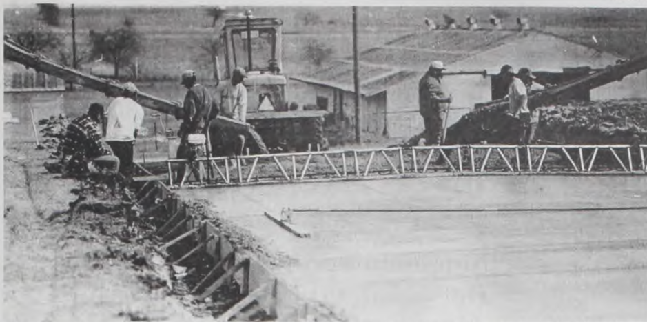
Major concrete construction is underway at Sacred Heart Cemetery as the second phase of the expansion project, the driving surface, is built. The parish has been saving for many
