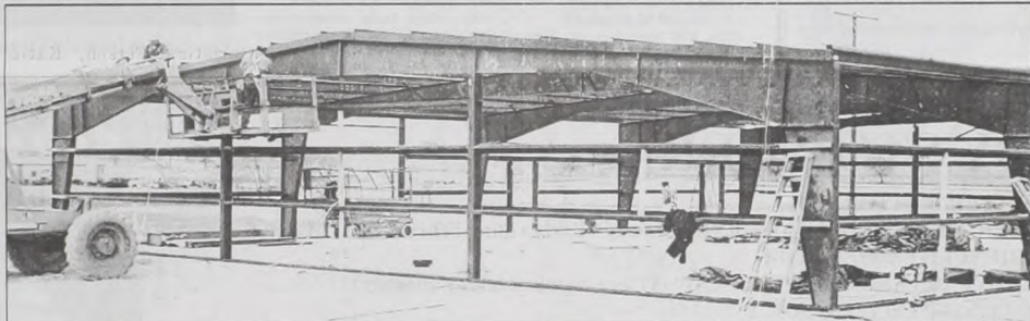
Work progressed quickly on the new athletic/maintenance building for Muenster ISD. Only a frame last week, the building is now in the dry.
