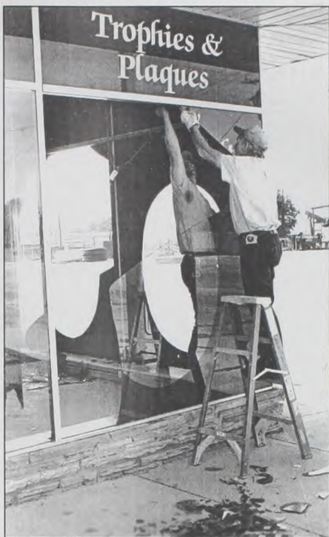
Workmen remove remaining broken glass from two large plate glass windows at Unique Images Friday morning after Thursday night's storm damage. Dave Fette photo
