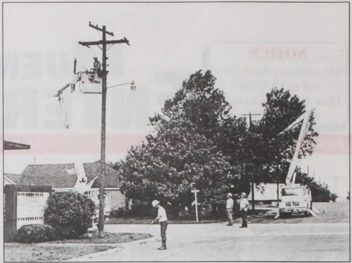
OnCor electrical crews were in Muenster early Friday morning after strong winds during the night caused damage to power lines. Workers return the lines to the poles on East First Street after large pieces of roofing were torn off the Frybrant building. Janie Hartman photo
