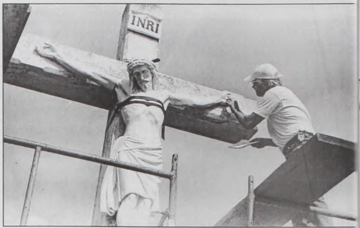
Rick Bennett of Special Stone Installation of Dallas makes repairs to the statue in Sacred Heart Cemetery. Vandals recently broke both hands and Christ's feet. The majority of the pieces were found and repairs were made. The Crucifixion Group was donated to the parish by Joseph and Mary Kleiss in 1917. Bennett will complete the repairs with a fresh finish to the entire monument. Janie Hartman photo
