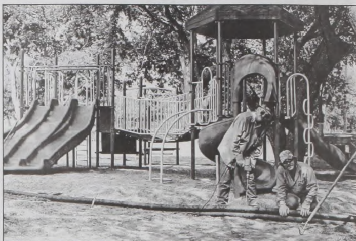
Muenster City employee Terry Stewart, left, and David Dittfurth install 4x4 Rumber border material around the new playground equipment in the municipal park Tuesday. Rumber Material, Inc. donated the border beams. The area around and under the play set is covered with eight inches of pea gravel. Dave Fette photo
