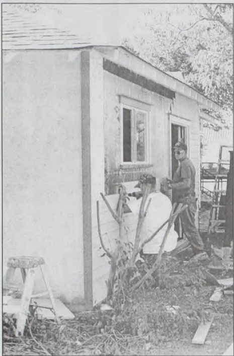
Remodeling of the Ben and Aggie Seyler Muenster Museum continues. The project includes closing in the breezeway and repairs to the garage. Improvements will increase display space and allow more exhibits to preserve history and share with the community. Janie Hartman photo
