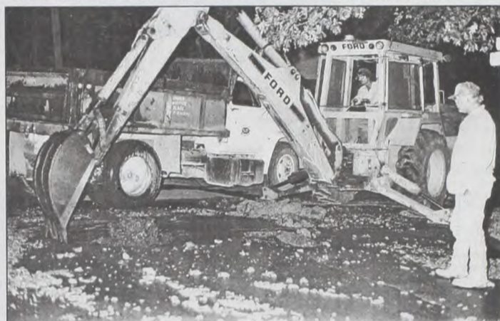
City employee David Dittfurth operates the backhoe under close monitor by Terry Stewart at the intersection of Hickory and Second Streets last Thursday night. City manager Linda Webb, water department manager Chris Yosten and the city crew plus helpers had to deal with a break in a six-inch water main under the street. The gusher broke through the surface and quickly drained out to Highway 82. Yosten and company had to dig out the hole, about 4 feet wide and six feet deep, use two portable pumps to get ahead of the water flow, then get a band clamp around the hole with water flowing. They filled the hole with sand and crushed rock. Time elapsed: 4 hours. The clamp is good for the life of the cast iron pipe. Dave Fette photo
