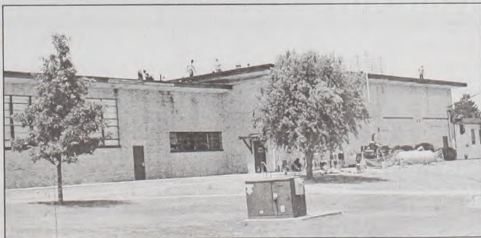
Repairs and improvements to the Muenster ISD campus buildings are in full swing in an attempt for completion before the August school bells ring. Watch next weeks Muenster Enterprise for an update on the progress of the construction. Janie Hartman photo
