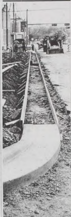
Work crews prepare to pour the curbing on the first block of Main Street after tearing out the week-old curb. According to Wayne Bell, area engineer for the Texas Department of Transportation, the curbs had the "wrong angle" for drainage. The crew laid the curbs tilted "down" and should have an upward tilt so the water runs down the curb and not the street, washing into the "hot mix crack." Janie Hartman Photo
