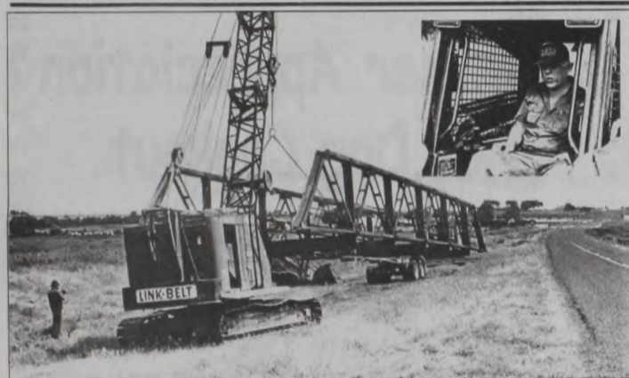
The old steel bridge that spanned Elm Creek just south of Lindsay beside Farm Road 3108 was removed Wednesday. Billy Lemons (inset) of Lemons House Moving, Whitesboro says the frame measured 18feet, 9 inches wide and 100 feet, 6 inches long. Lemons says he probably has the bridge sold to the Tribute Golf Course in The Colony, Texas.
