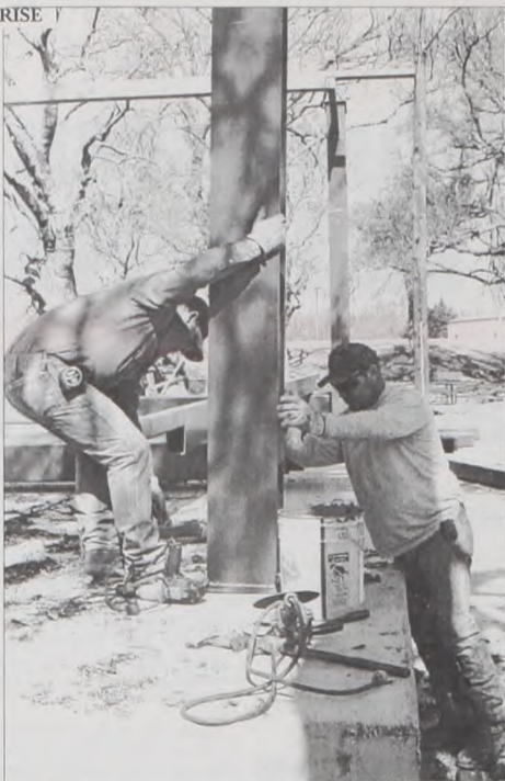
The weather was great Wednesday for David and Shawn Flusche of Structures, Inc. to begin construction of the framework for the performing arts stage in Muenster's City Park. Dave Fette Photo
