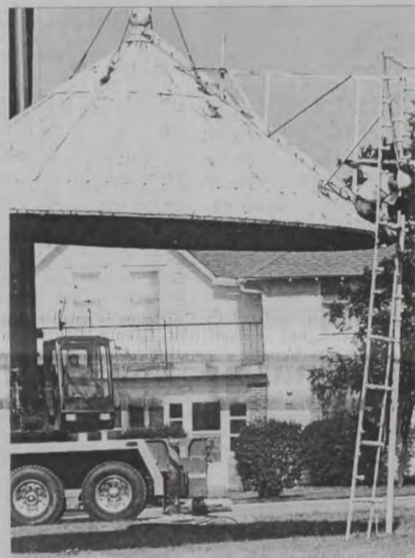
Workers lower the top of the old water tower during dismantling last month. The roof may be used in the construction of a gazebo in one of the city's parks. Janie Hartman Photo
