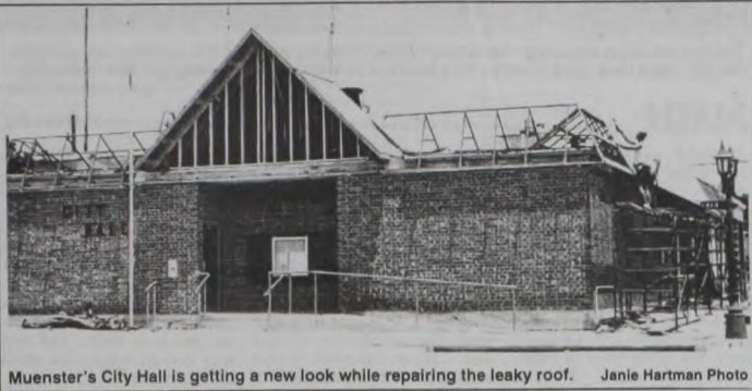
Muenster's City Hall is getting a new look while repairing the leaky roof. Janie Hartman Photo
