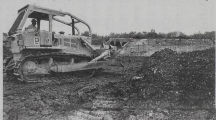
The concrete trestle on the old railroad right-of-way stands in lonely defiance to the huge bulldozer clearing the way for its removal from the Muenster Lake dam site. The 1929 date embedded in the concrete was cut away to save for display. Dave Fette photo
