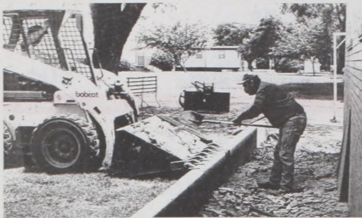
Doug Martin and Shane Huchton of Huchton Construction (in Bearcat) clear away the sidewalk at the northeast side of Sacred Heart Church. The crumbling walkway will be replaced, including better level for drainage. Janie Hartman Photo
