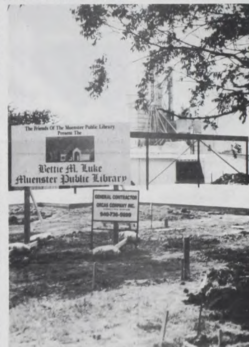
The new Muenster Public Library showed a sign of going up Tuesday when the first of the frame work could be seen standing
