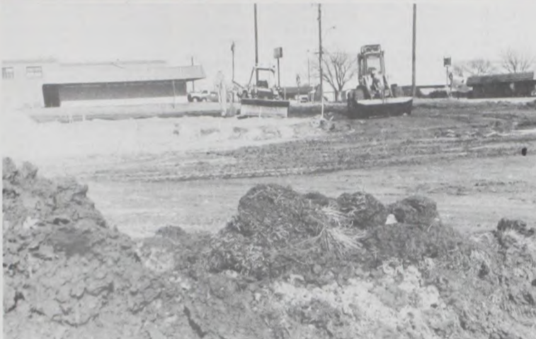
Turning the dirt at the future site of Muenster's Sonic Drive-In continues at the corner of South Mesquite and Division Streets. The facility will include 24 car stalls at the drive-in and two ordering stations under a covered patio. Manager Kenny Jones hopes to open in March and could employ 40-45 people. A backhoe accident at the site last Thursday ended on a good note, the worker is okay and recuperating at home. Photo by Janie Hartman
