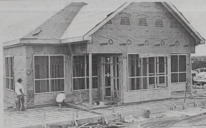
Work is progressing swiftly on the new post office being built in Muenster. L & M Construction of Kellyville, Oklahoma is the contractor. Top photo taken Saturday shows completed framework approximately one week after the slab was poured. The bottom shows progress done on the building by Tuesday morning. Staff photos
