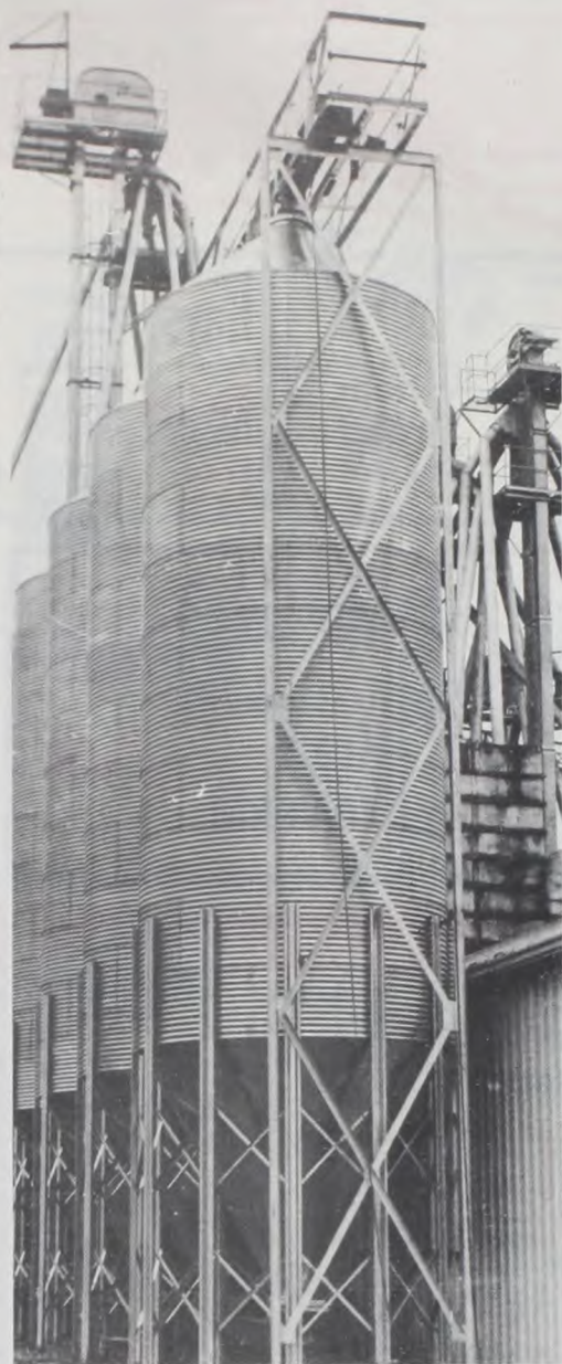
Work continues at Tony's Seed and Feed, South Main Street in Muenster, with the addition of five 2,800 bushel hopper bins. The added storage will be used for raw ingredients or unfinished feed and should be completed in a couple of weeks.
