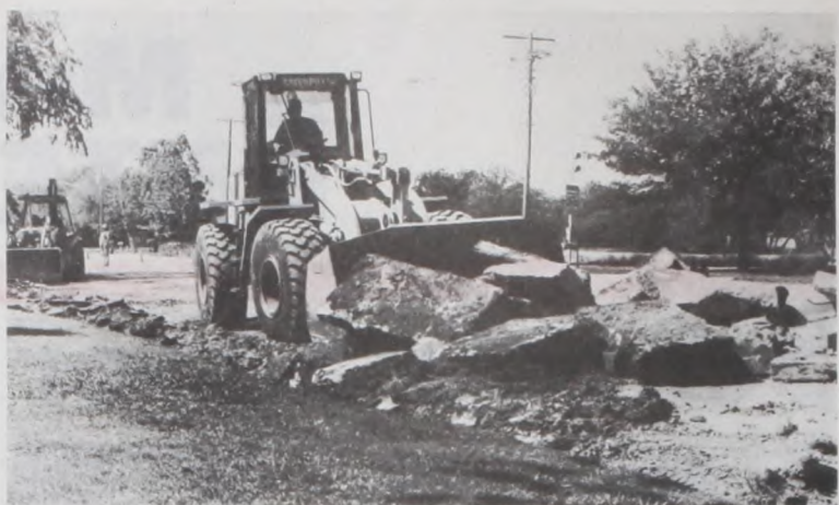
Work began this week on a job long overdue — the re-curb-ing of Main Street north of Seventh. The old broken, sunken curb was removed on both sides of the street in preparation for new curbs, later to be followed by a new street surface. Photo by Janie Hartman
