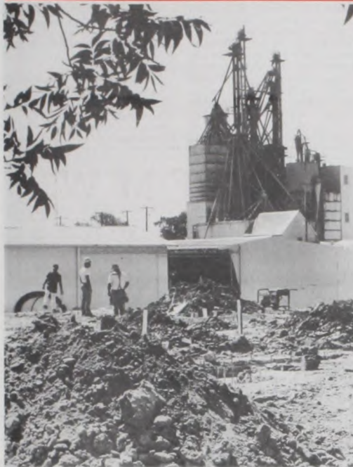
With the completion of "dirt work" at the site of the future Muenster Public Library, workers prepare the base for the pouring of the cement slab. The plans for a new library building have been in the making for over six years. With the financial support from "friends" of the library, the project is now becoming a reality. Photo by Janie Hartman
