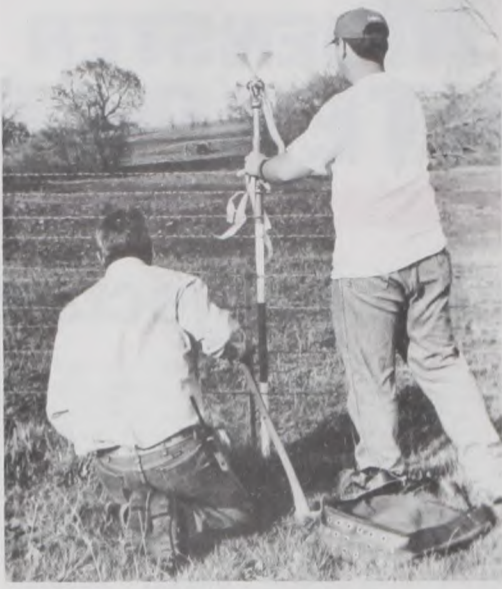
Surveyors were staking out the perimeter this week for core drilling at the future site of Muenster Lake. Core testing will classify the soil to be used in building the lake dam. Victor Rice and Todd Solley of Rice Inspection, Inc. of McGregor, Texas mark the location as Trenton Rice, in the distance, takes the elevation readings. Janie Hartman photo
